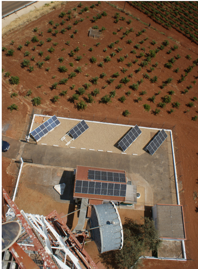
Photovoltaic panels were installed at the communications centre «ALMENDRALEJO» (BADAJOZ), the first communications centre of the Spanish Armed Forces to be powered by this system.
