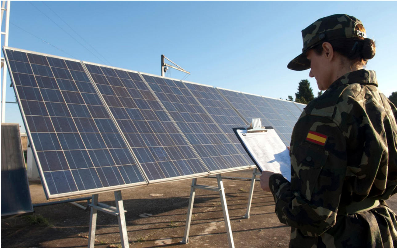
The use of clean energy sources such as solar energy is becoming increasingly common in the Ministry of Defence's facilities.
